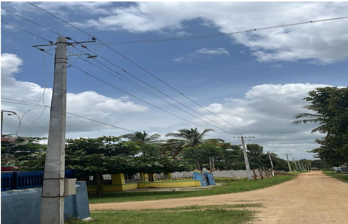
Street lights installed at the centre of I-village near community hall.
