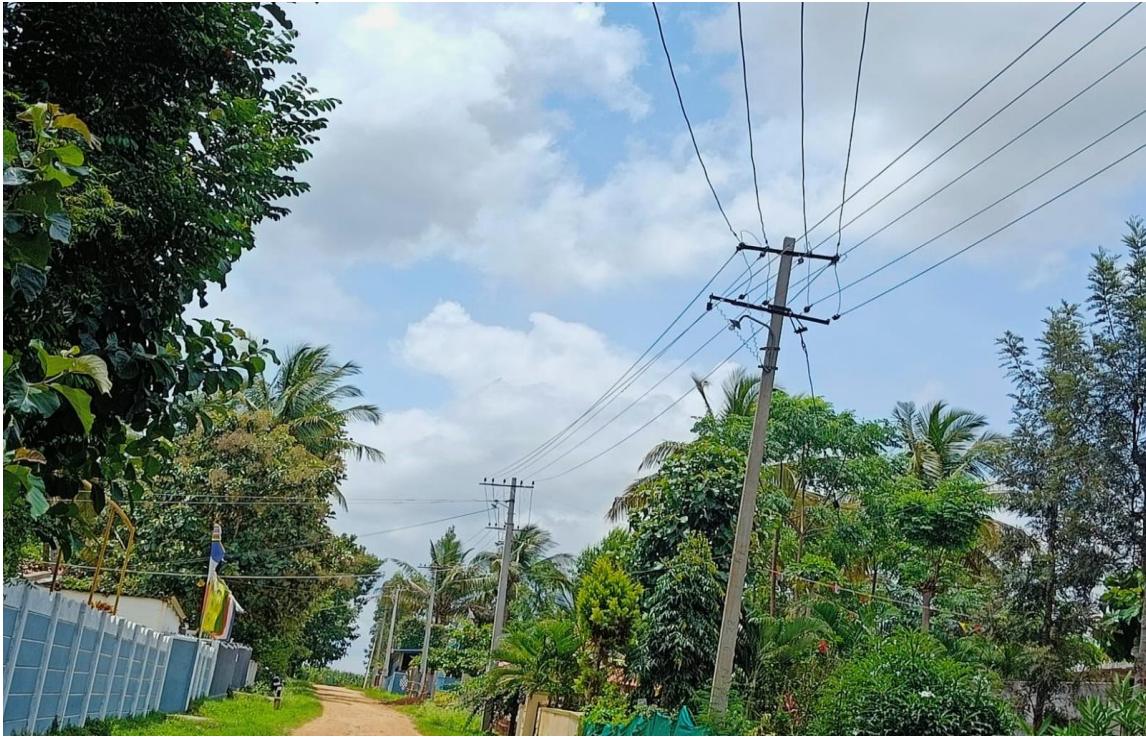
Street lights installed around the residents.
