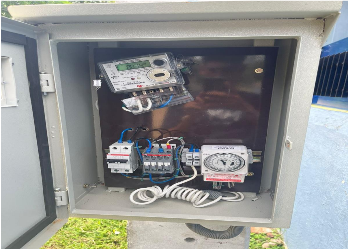
Electricity meter with time for street light.
